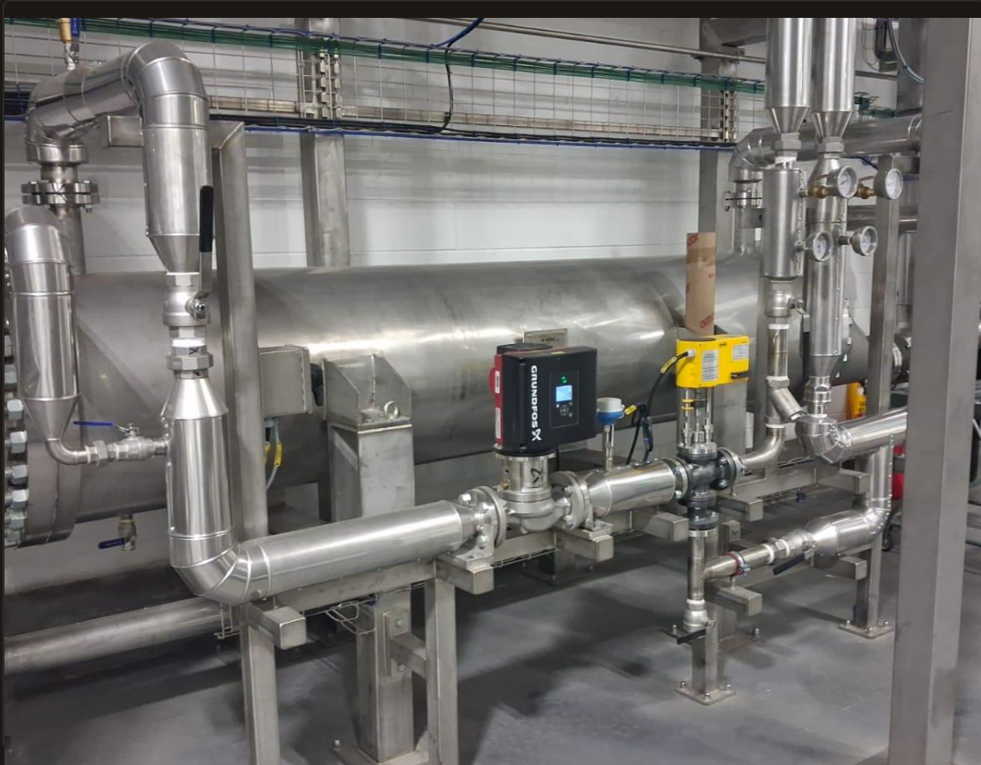
HEAT EXCHANGER STATIONS
